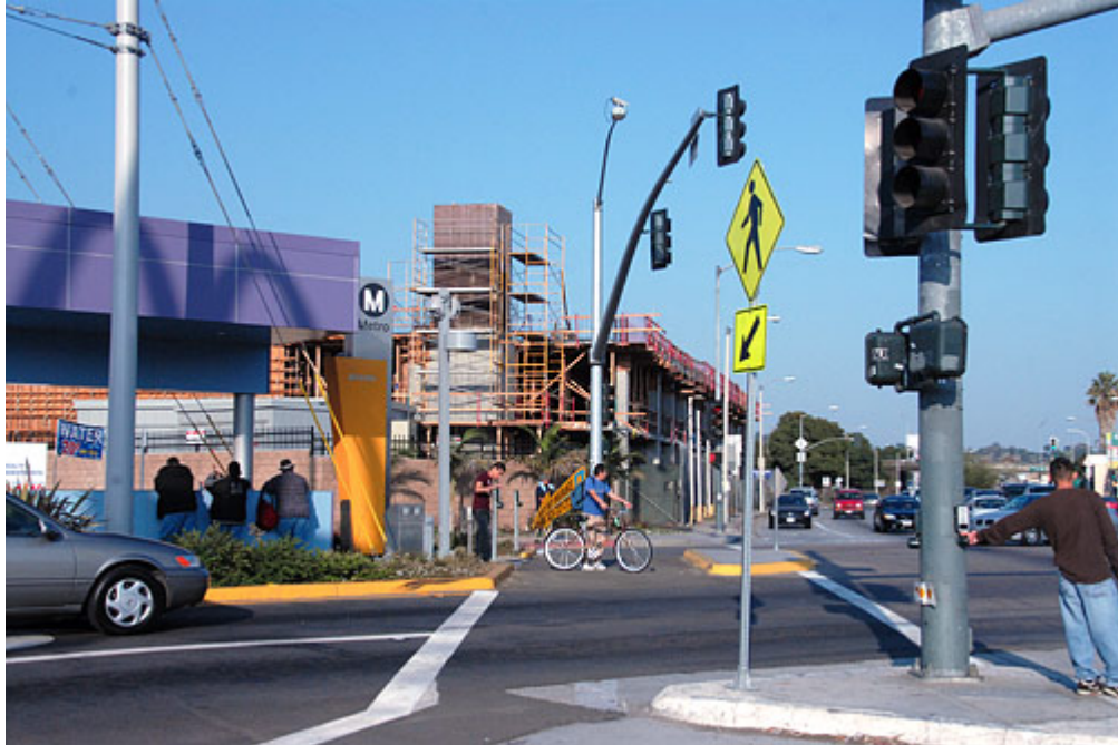
At the east end of the Gold Line, a parking structure will soon provide some 280 parking spaces for Metro riders willing to park their car and take the train the rest of the way.
