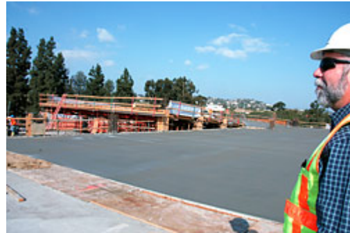
Resident Engineer Matt Gallagher watches as crew lays down last 320 yards of concrete deck to complete top level.
